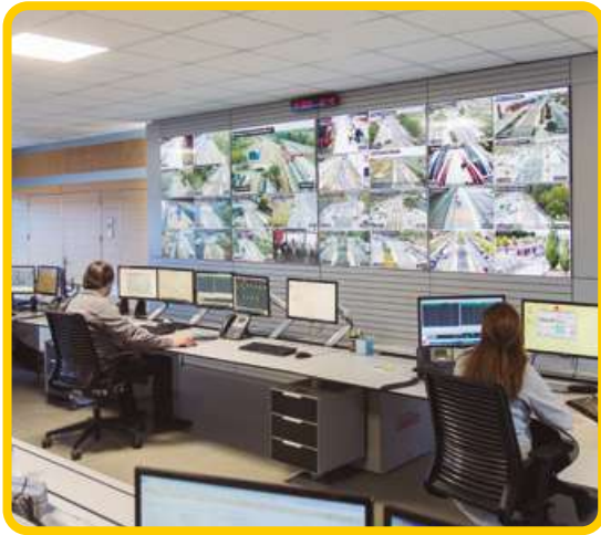
CCC – Central Control Centre
